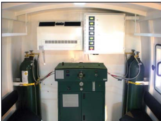
CO 2 scrubber with oxygen cylinders *Optional air conditioner & monitoring system
